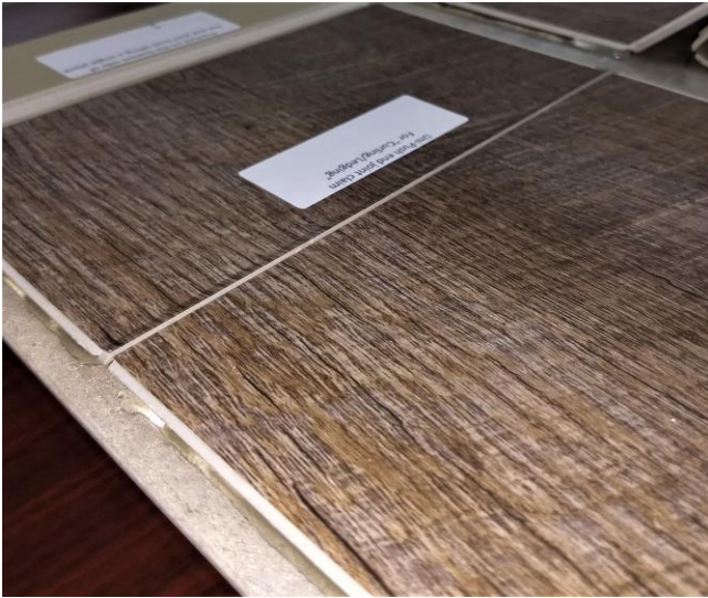
Looking into the raised end of the damaged Uni-Push end joint.
