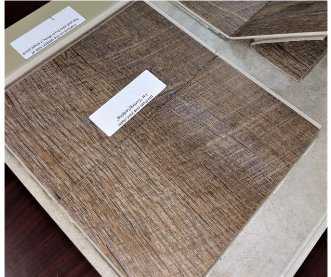
Looking down towards the raised end of the damaged Uni-Push end joint.
